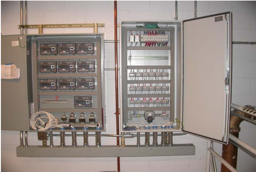
Johnson Controls and Main Emacx Panel Zuckerman Building
