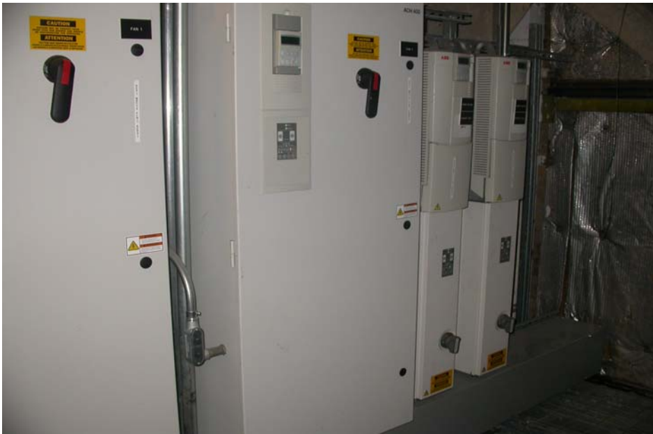
Installed 250Hp VFD for Air Handlers
