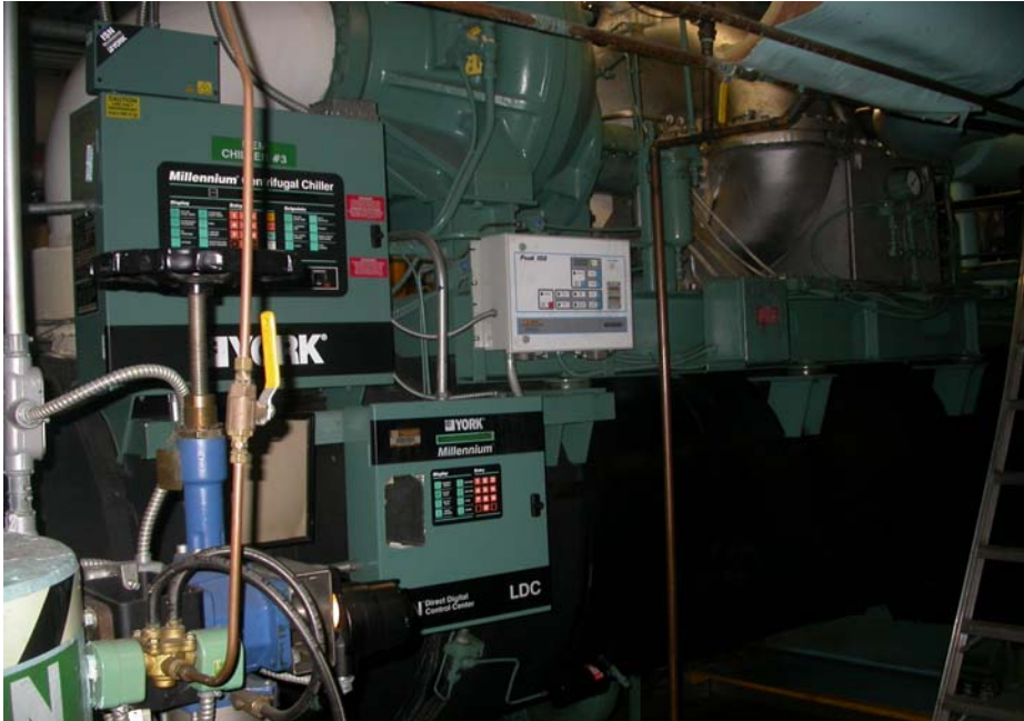
Chiller Integration through Remote Chill Water Reset for DR
