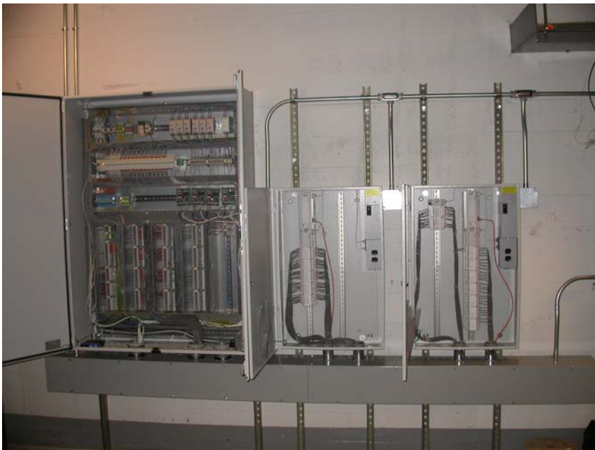
Main Emacx Panel EMA and Siemens I/O Panel
